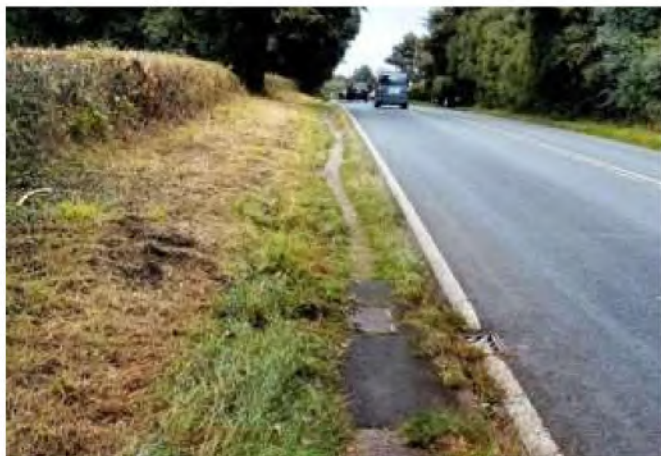
Fig 62. A poorly maintained footpath alongside the A44 1 at Hopwood
