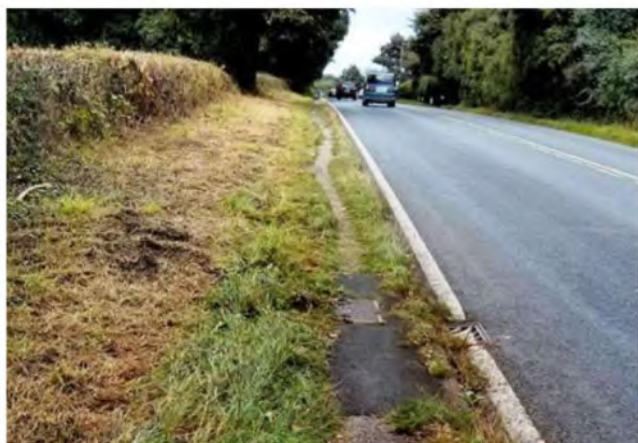
Fig 11. Public highway footpath, too narrow and too close to the main highway
