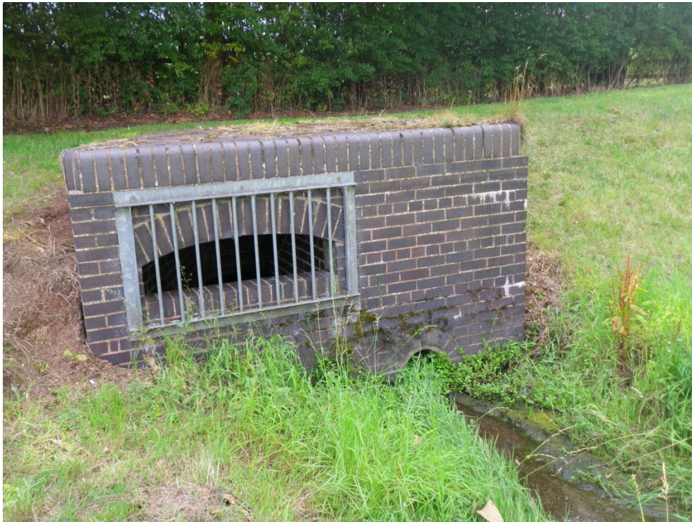
Photograph 18 - Attenuation area control structure, Church Road, Webheath
