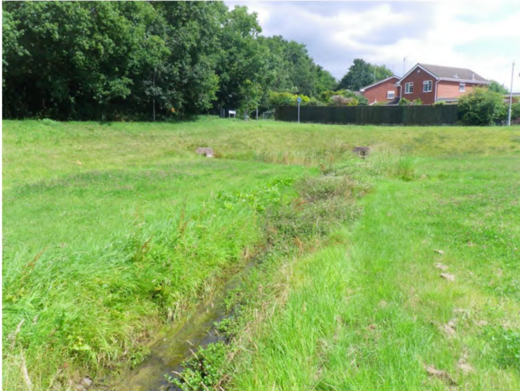
Photograph 19 - Attenuation area control structure, Church Road, Webheath
