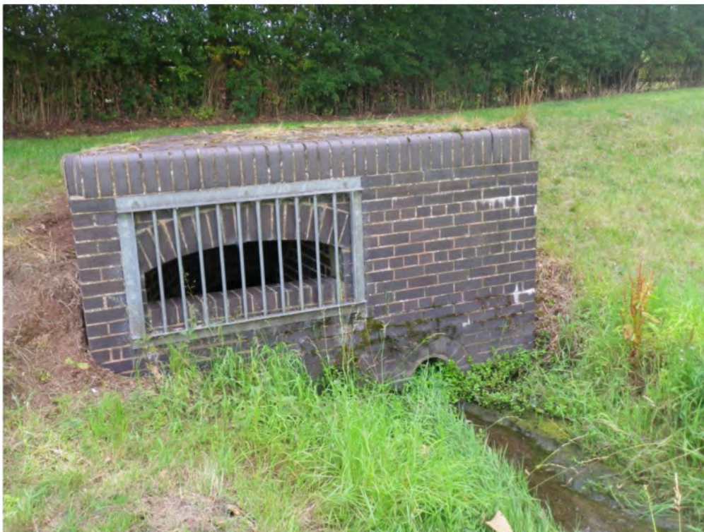
Photograph 18 - Attenuation area control structure, Church Road, Webheath
