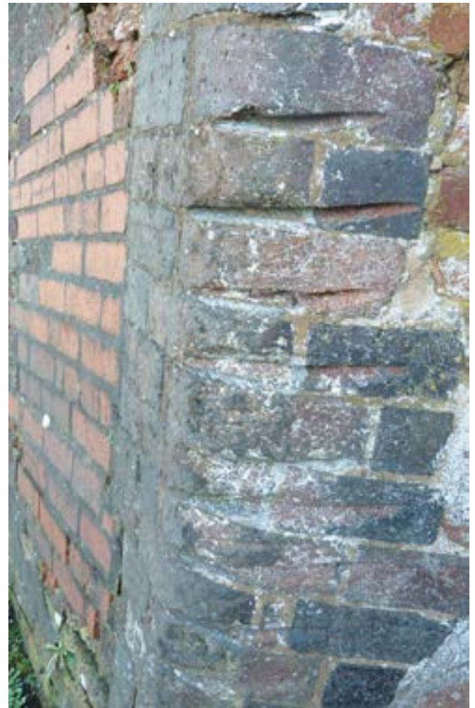
Rope marks on a bridge wall
