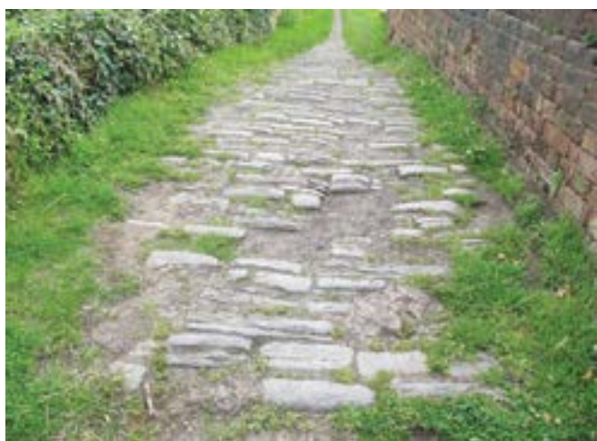
The canal arm bridge at the old Salt Works site with the setts before their removal
